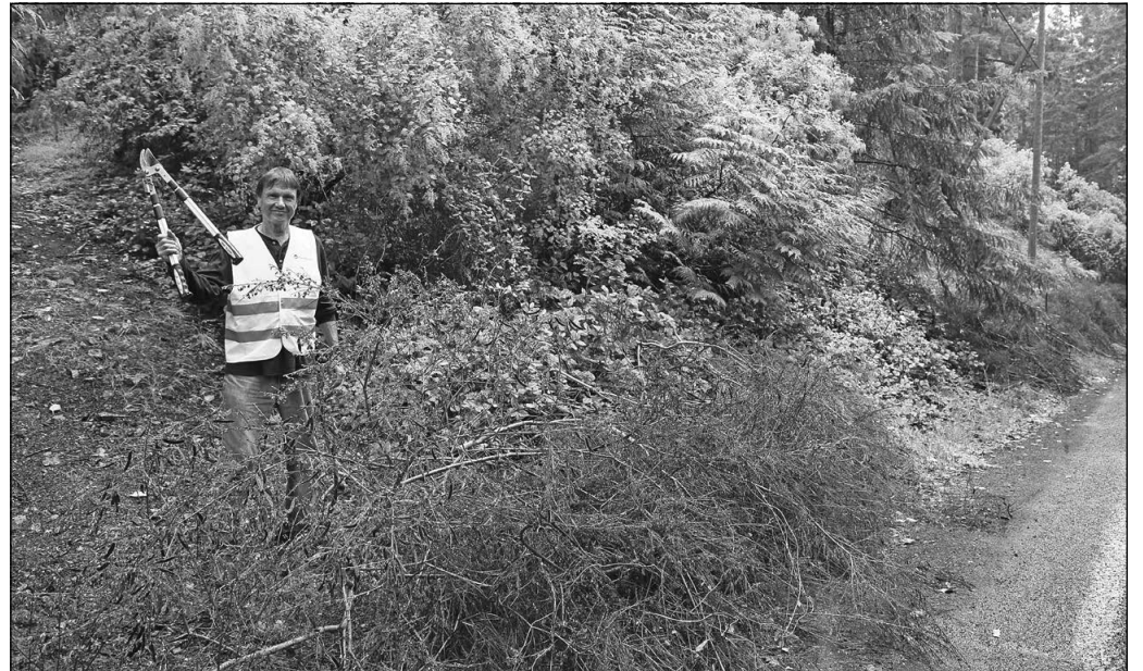
Lyle Petch works to clear more Scotch broom from the side of Old Scott Road.
