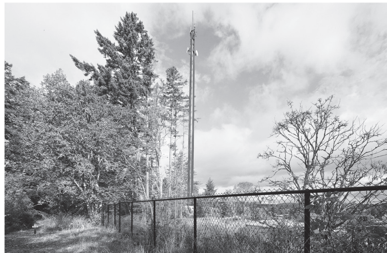
PHOTO COURTESY CREST An example of a typical CREST VHF monopole, as seen at the View Royal Fire Hall.
