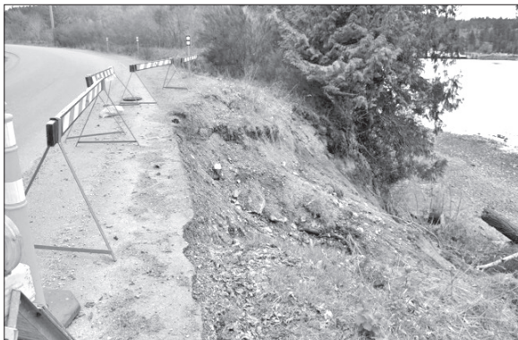
Safety barriers at the site of a major washout on Isabella Point Road. PHOTO BY DAN DICKMEYER
