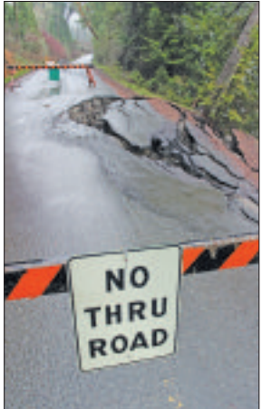
PHOTO BY JEN MACLELLAN North Beach Road was closed after part of it washed away in February.
