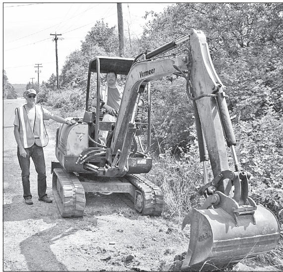
Volunteer project manager Richard Shead, left, and contractor Chris Magnus begin Rainbow Road path extension work.
