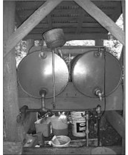
Fuel stand on Russell Island where fuel had been stored in the past.
