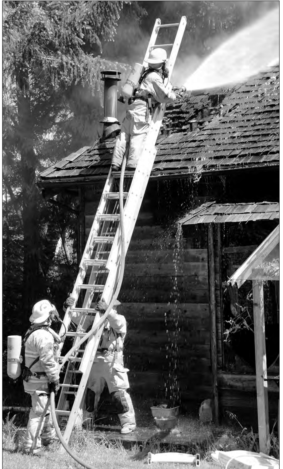
This structure fire on Byron Road was just one of several fires fought by local Fire-Rescue crews in the spring of 2010.
