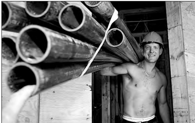
12:45 pm: Aidon Morris carries pipes at a Ganges construction site. Photo by Derrick Lundy.
