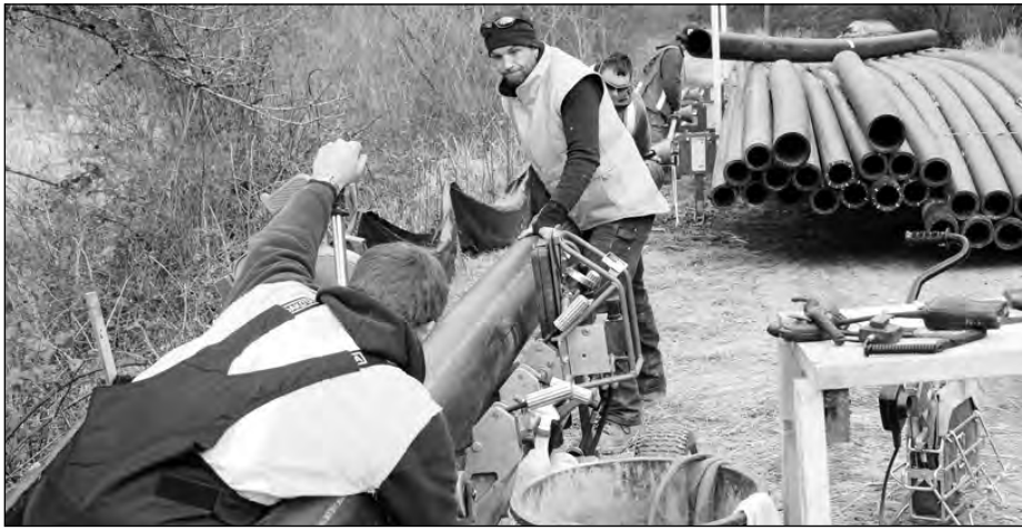
Rick Mayes and Mike Shanahan lay out pipe at St. Mary Lake.
