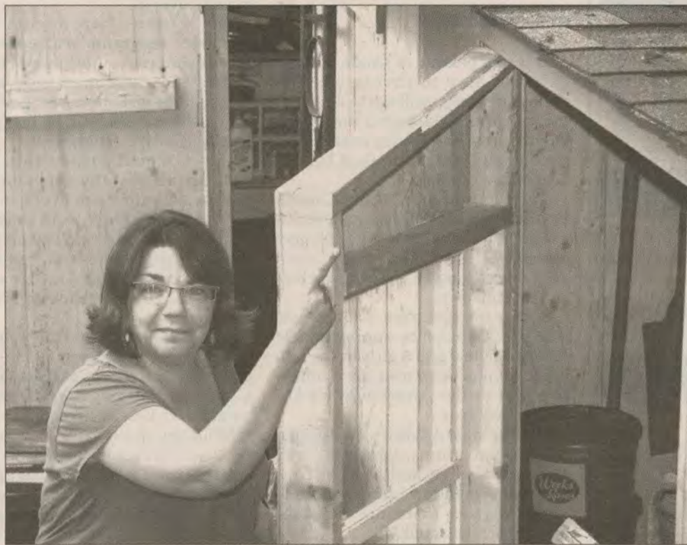
Chris Leichner points to a botched door installation job on her wood shed.
