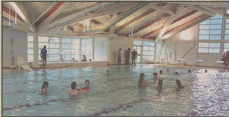
Workers look on as a few lucky high school students provide the waves for testing the new pool systems.
