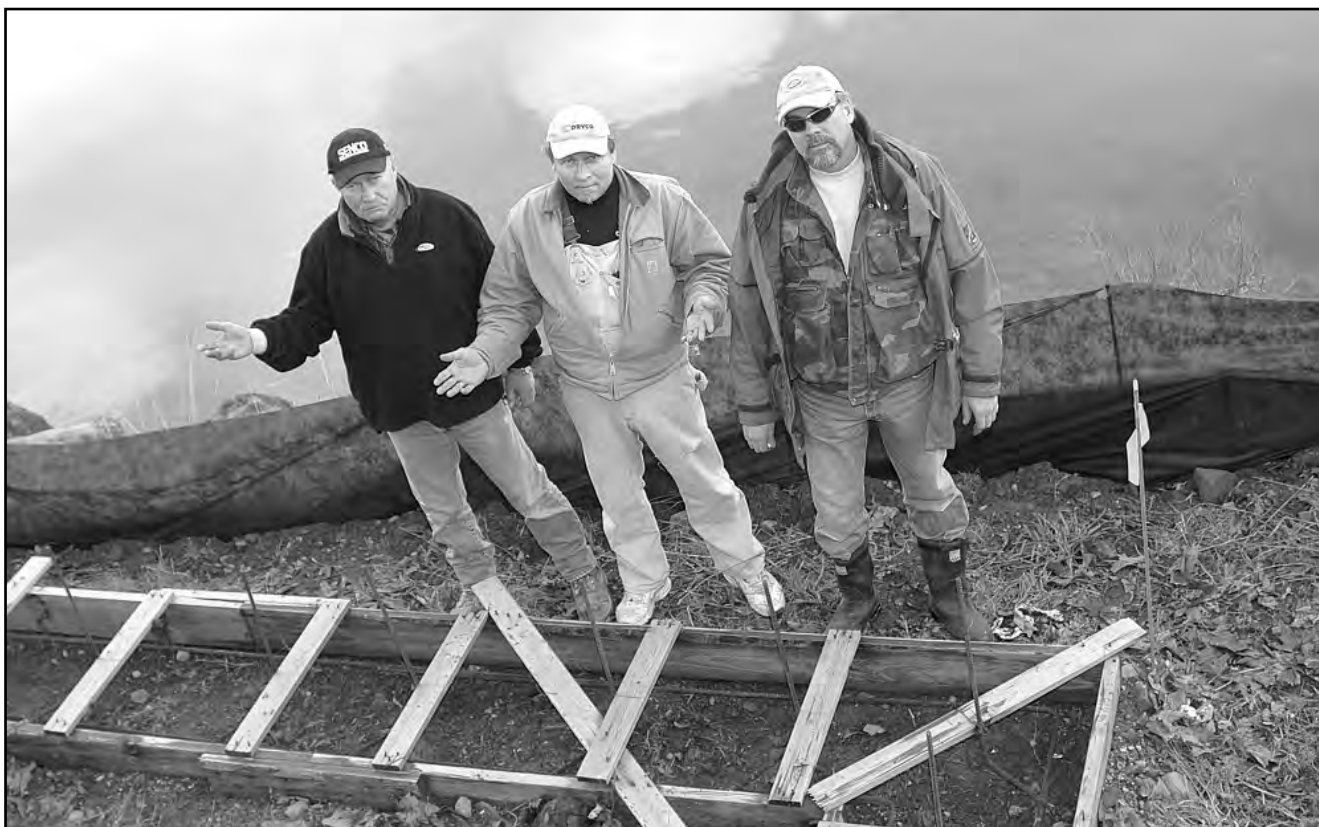
NO GO: From left, Barry Long, Peter Orel and Ken Prebski of Bear Contracting are all ready for a cement pour at Ganges Marina. A stop work order brought the pour to a halt. Photo by Derrick Lundy
