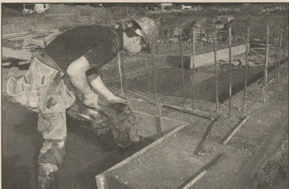
FINE FORMS: Ben Wright tears apart forms from the first concrete pour at Salt Spring's indoor pool construction site. Photo by Derrick Lundy
