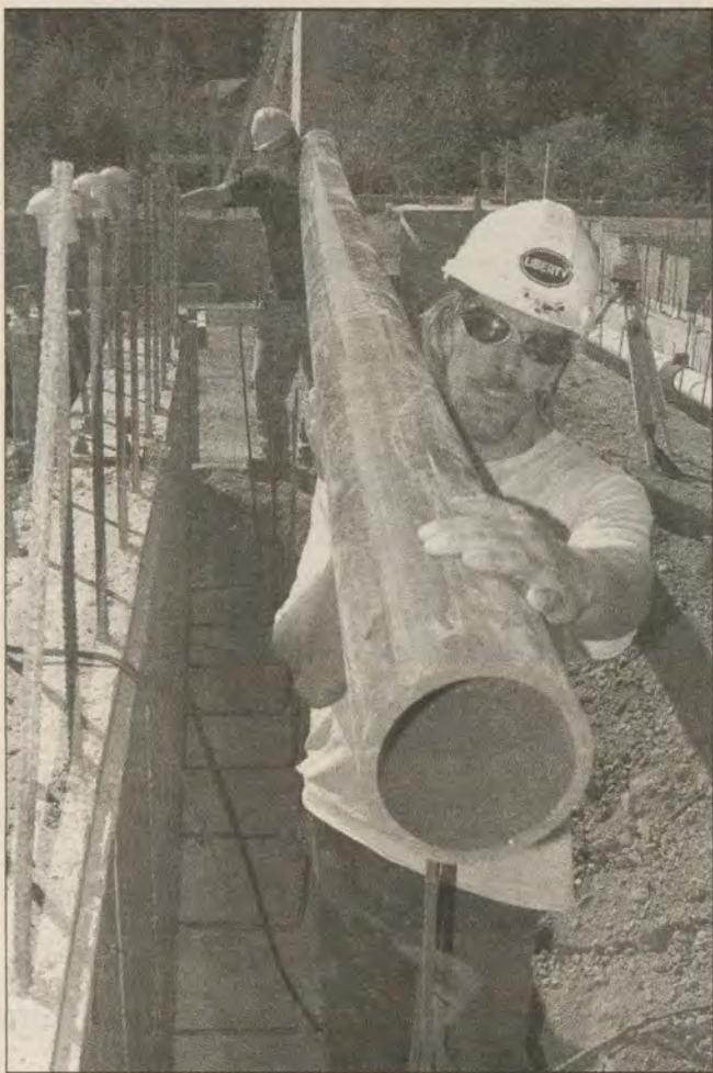
POOL PRECISION: Marc Ponton, front, and Blair Darcy carry pipes to plumb the hot tub at the Rainbow Road pool construction site. Photo by Derrick Lundy
