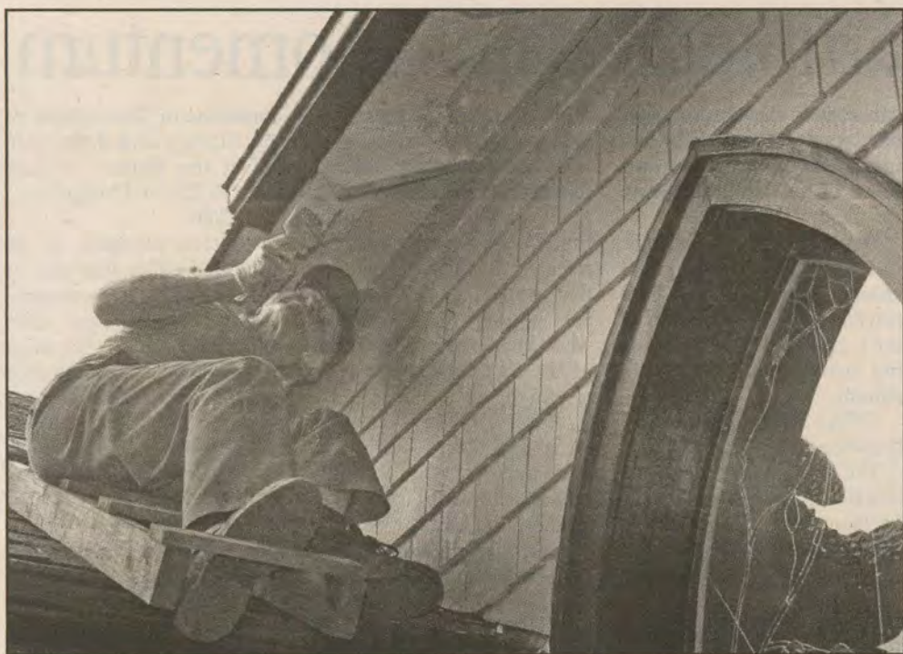
COLOUR TOUCH UP: Gordon Cartwright adds a fresh coat of paint to the underside of the roof at Ganges United Church. Photo by Derrick Lundy
