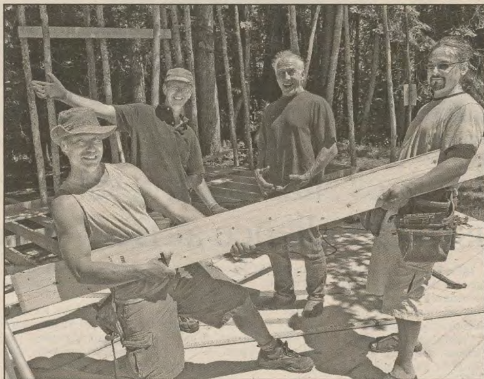
CENTRE STAGE: From left, John French, Vaughn Fulford, Scott Hylands and Richard Williams use some theatrical flourish as they work on construction of a theatre in Mouat Park.
