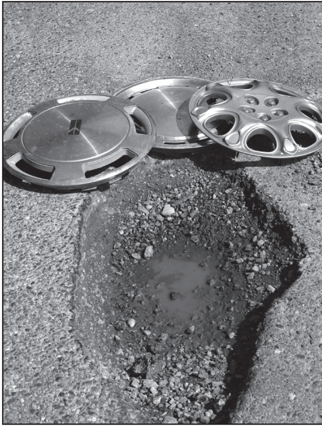
HUBCAP HEAVEN: A hubcap shrine was recently set up next to this eight-inch-deep pothole on Mansell Road. Photo by Derrick Lundy
