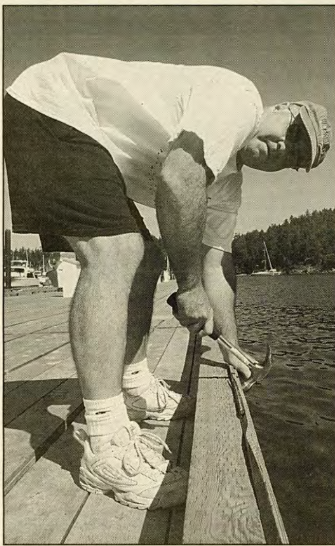
HAMMERING AWAY: Ganges Marina project manager Robyn Kelln hammers a board on the outside edge of the marina's breakwater Tuesday to prohibit boaters from tying up in those spots. The move puts the marina in compliance with its Trust development permit and water lease restrictions.
