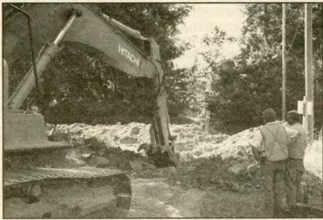
WORK IN PROGRESS: Site servicing work undertaken by Spencer's Excavating crews is well underway at the Rainbow Road rec facility site. Regardless of whether an indoor or outdoor pool is built on that spot, water and sewer lines are being installed now. Photo by Dave Gibbon
