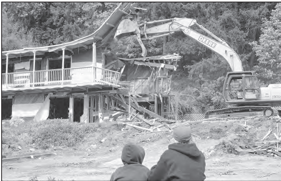
GOING DOWN: Melanie and Jordan Berry watch Monday afternoon's demolition of the Beachcomber Motel on Vesuvius Bay Road. Melanie said the old motel had been a landmark in the area since she was born over three decades ago.
