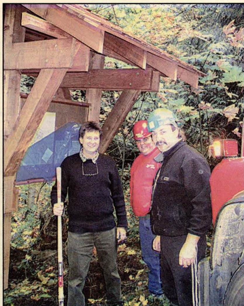
With help from JJM Contractors personnel, Channel Ridge Properties Ltd. Chair Kevin Thompson (left) has a look at the new information kiosks being installed last month at three entrances to the Channel Ridge trails. The trails are open to all members of the public daily from dawn until dusk and detailed maps are available for trail users at the kiosks.
