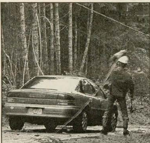
SHOCKING EXPERIENCE: B.C. Hydro linesman Don Fisher removes a power line that trapped two women in their car after a windstorm blew a tree across Channel Ridge Drive Friday morning.
