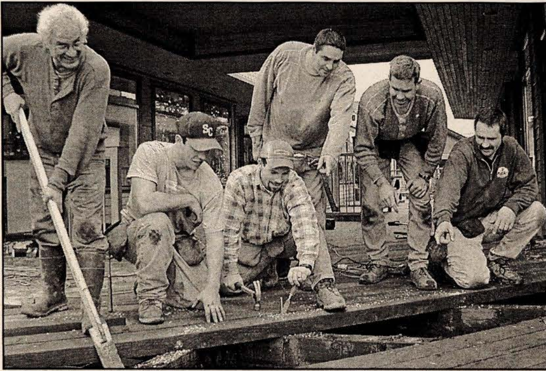
BOARD WORK: Rumour may have it that the W Huser & Sons Construction team is looking for a loonie dropped by Creekhous owner Leon Aptekman, but in fact, the boys were out in force replacing a portion of the walkway in the rain last week.
