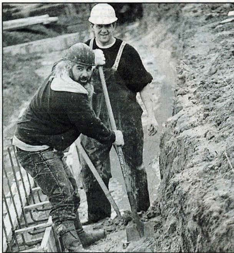
CLEANING UP: Ron Marks (front) and Dean Alexander get down to work Monday on the footings around the foundation at Ganges Village Market's new addition. Weekend rain filled up much of the footings with water and mud. Photo by Derrick Lundy
