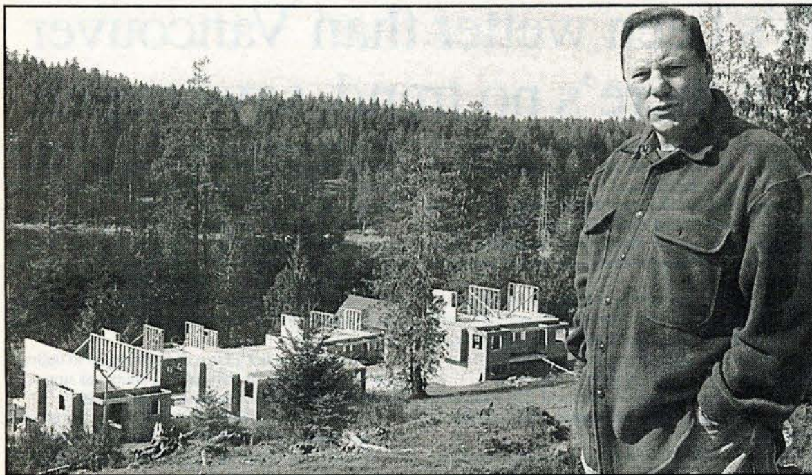
DREAMS FOR SALE: Developer Brian Hauff maintains a clear vision of his partially completed Salt Spring Island Village Resort project on Bullock Lake despite regulatory problems that stopped construction five months ago. Photo by Valerie Lennox
