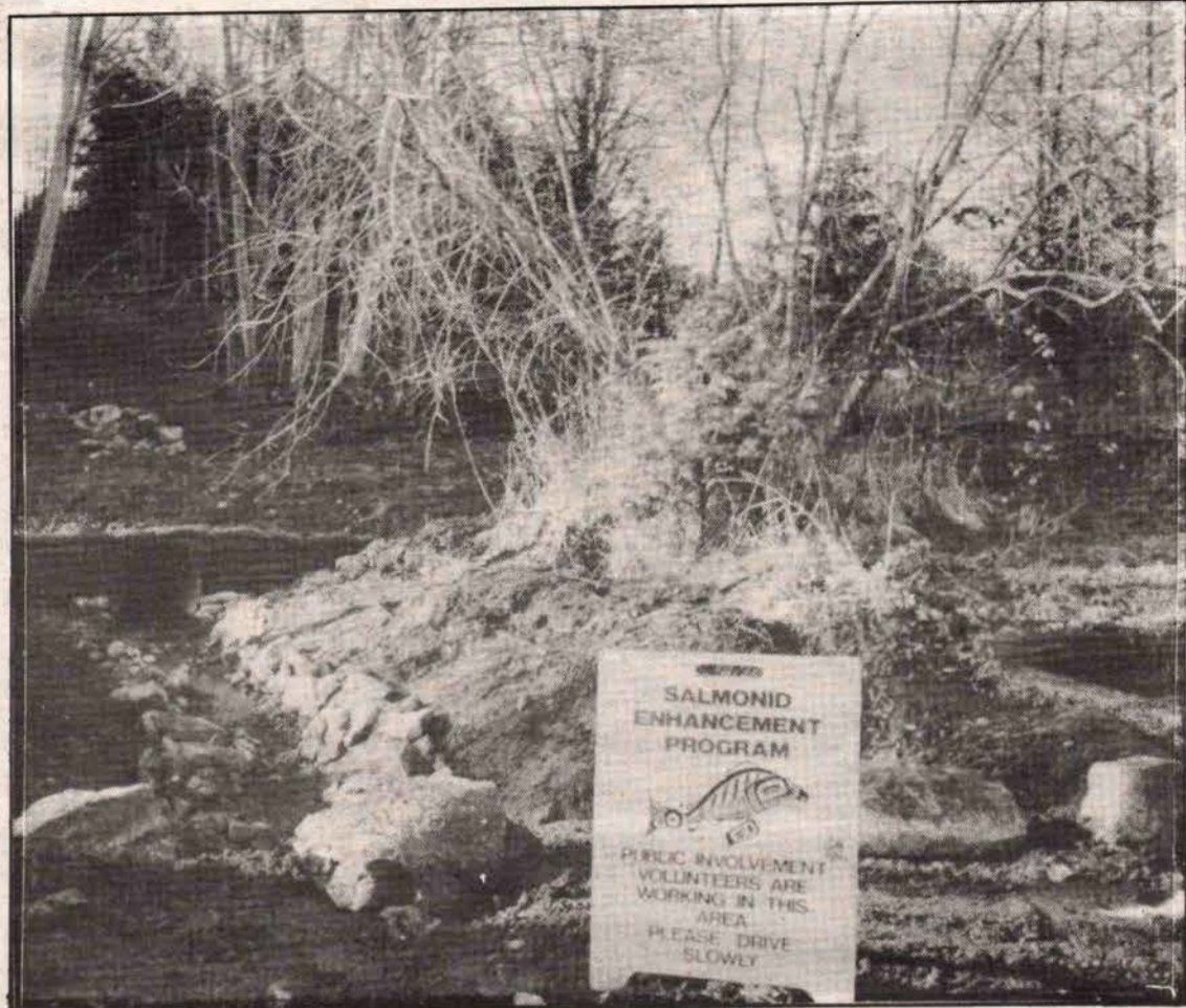
STREAM UNDER CONSTRUCTION: A sign marks a Salt Spring Island Salmon Enhancement Society project. Kathy Reimer
