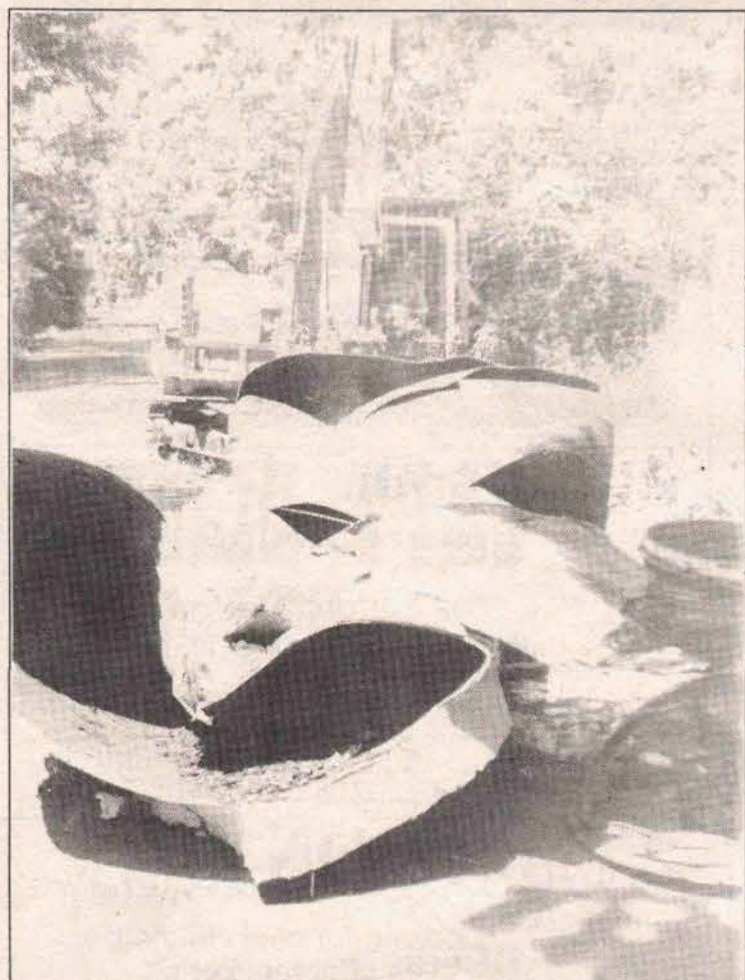
SCRAP METAL: The four large metal aerators in St. Mary Lake were hauled out of the lake Friday and broken up to be recycled. Ken Byron did the heavy work with his excavator, pictured here, while Ward Drummond hauled everything away.
