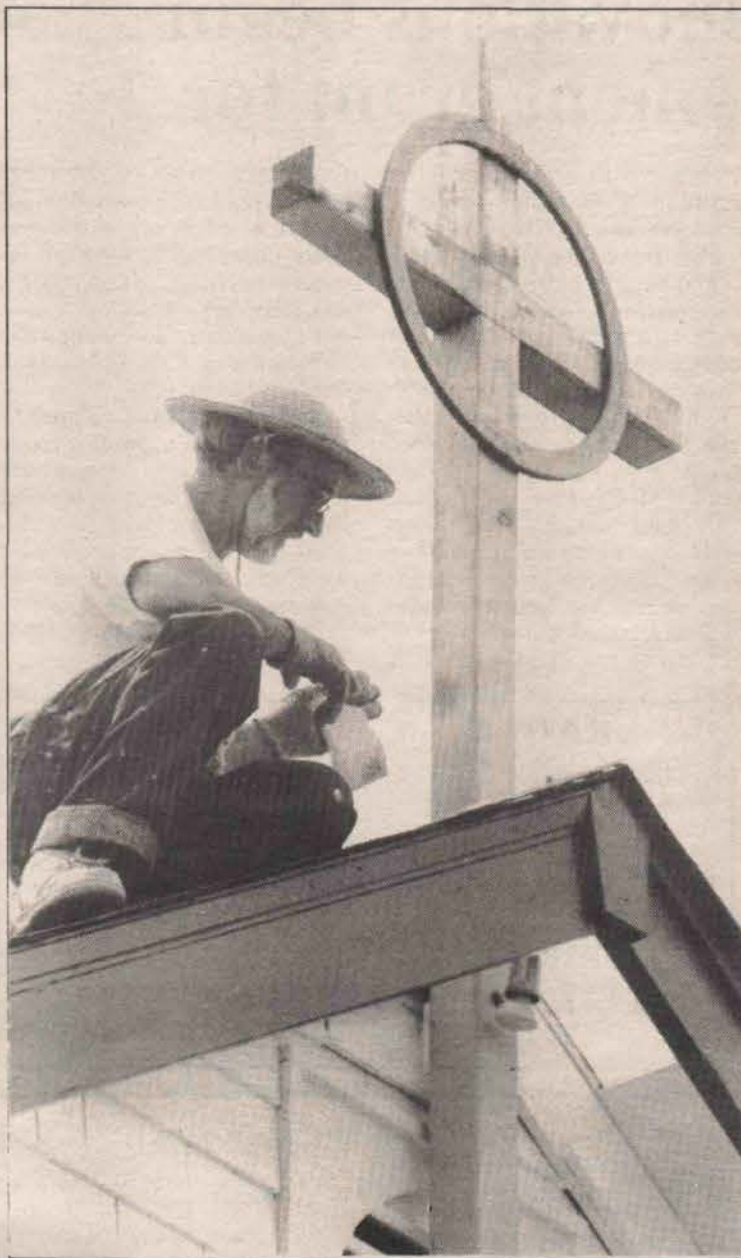
CLOSER TO GOD: If proximity to the heavens — and the cross atop Ganges United Church — puts one closer to God, then painter Tom Mitchell is right up there. Mitchell was working on the church last week, giving it a new look by painting the brown, shingled walls white.
