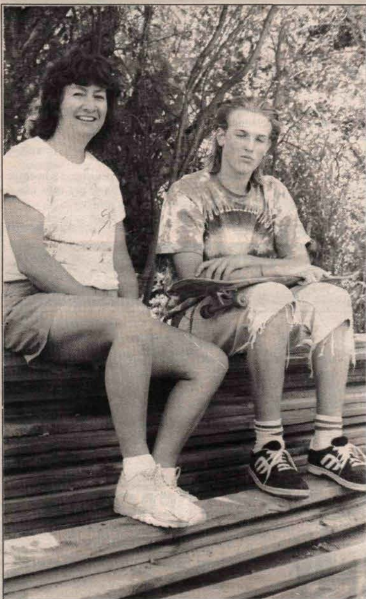
CLEAN-UP CONTINUES: Trish Nobile, left, and Dave Greig sit on a pile of re-usable boards taken out of the Core Inn on McPhillips Avenue. Preparations for renovation work continue with the help of Greig and Brett Gaylor, two students hired for the purpose.
