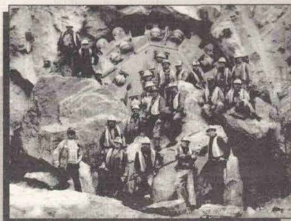
Rock and tunnel workers break through at the half-way point of the new KCP power tunnel (1991).
