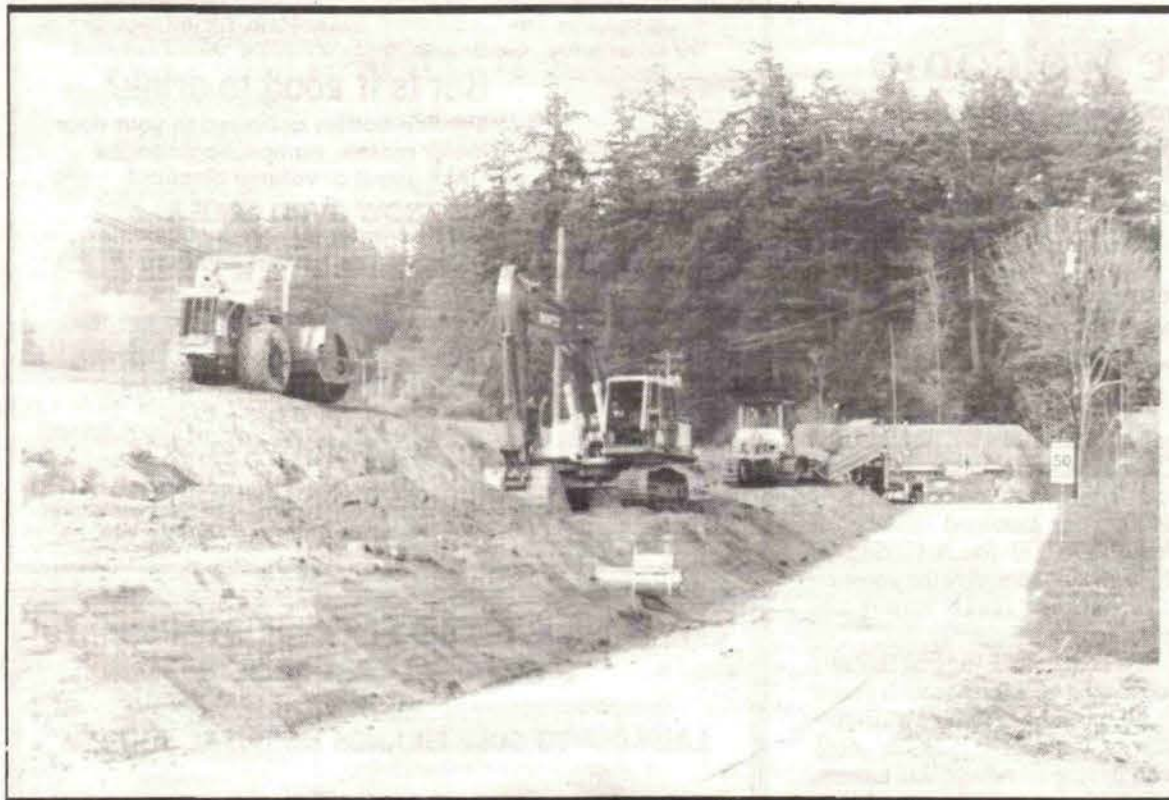
GOING UP: Roadwork near the Harbour House Hotel in Ganges has been steadily raising the level of Upper Ganges Road during the past two weeks. The steep grade at the intersection with Lower Ganges Road has been removed and the latter has been widened to accommodate a turn lane.
