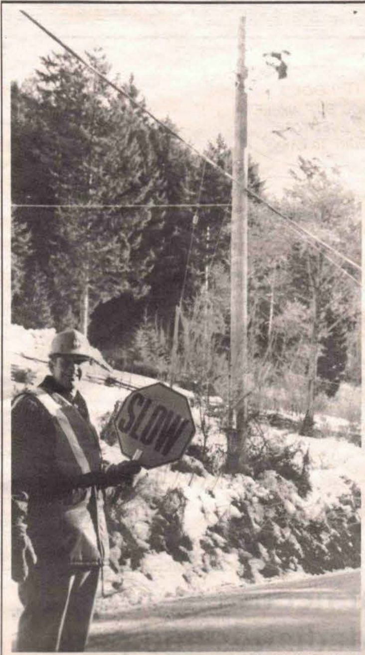
HIGH WIRE: B.C. Hydro crews were busy last week installing new wires on Cusheon Lake Road. Marvin Young slows down traffic while Pat Kelly does his work from the bucket.
