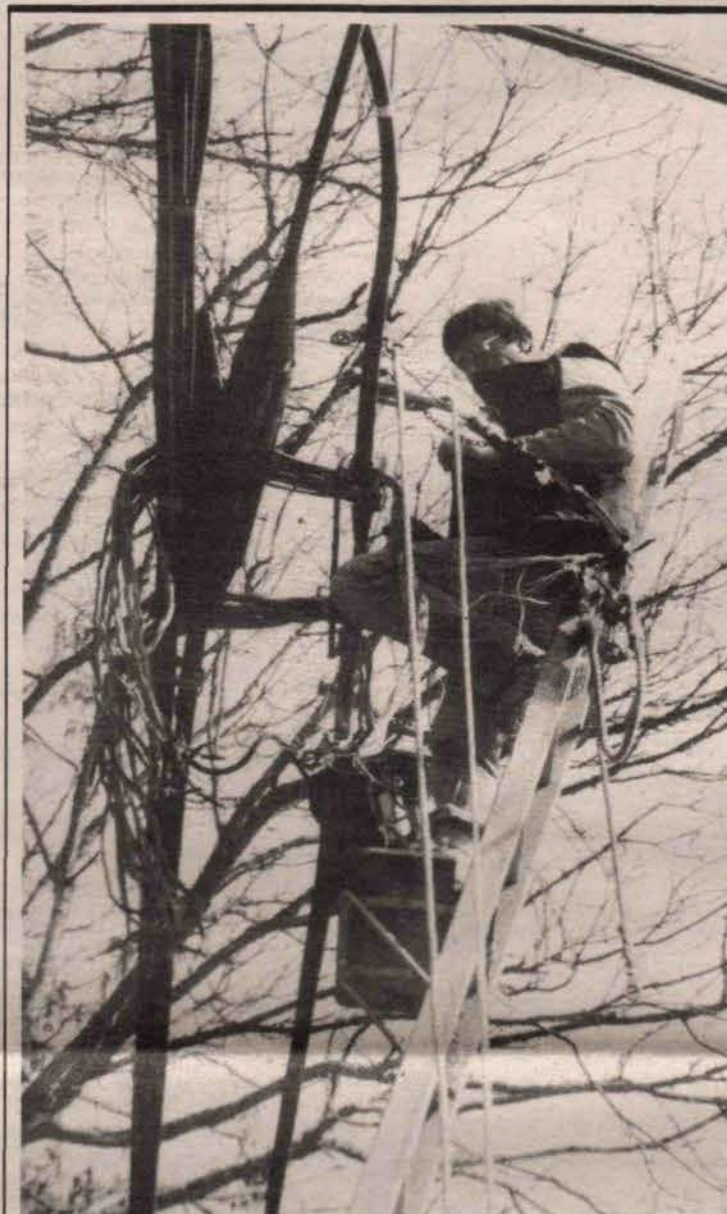
A SPLICE OF LIFE: A B.C. Telephone Company worker was busy splicing cables last week at the corner of Upper and Lower Ganges Roads. Recently laid underground cables on the west side of the road make the above ground cable unnecessary.
