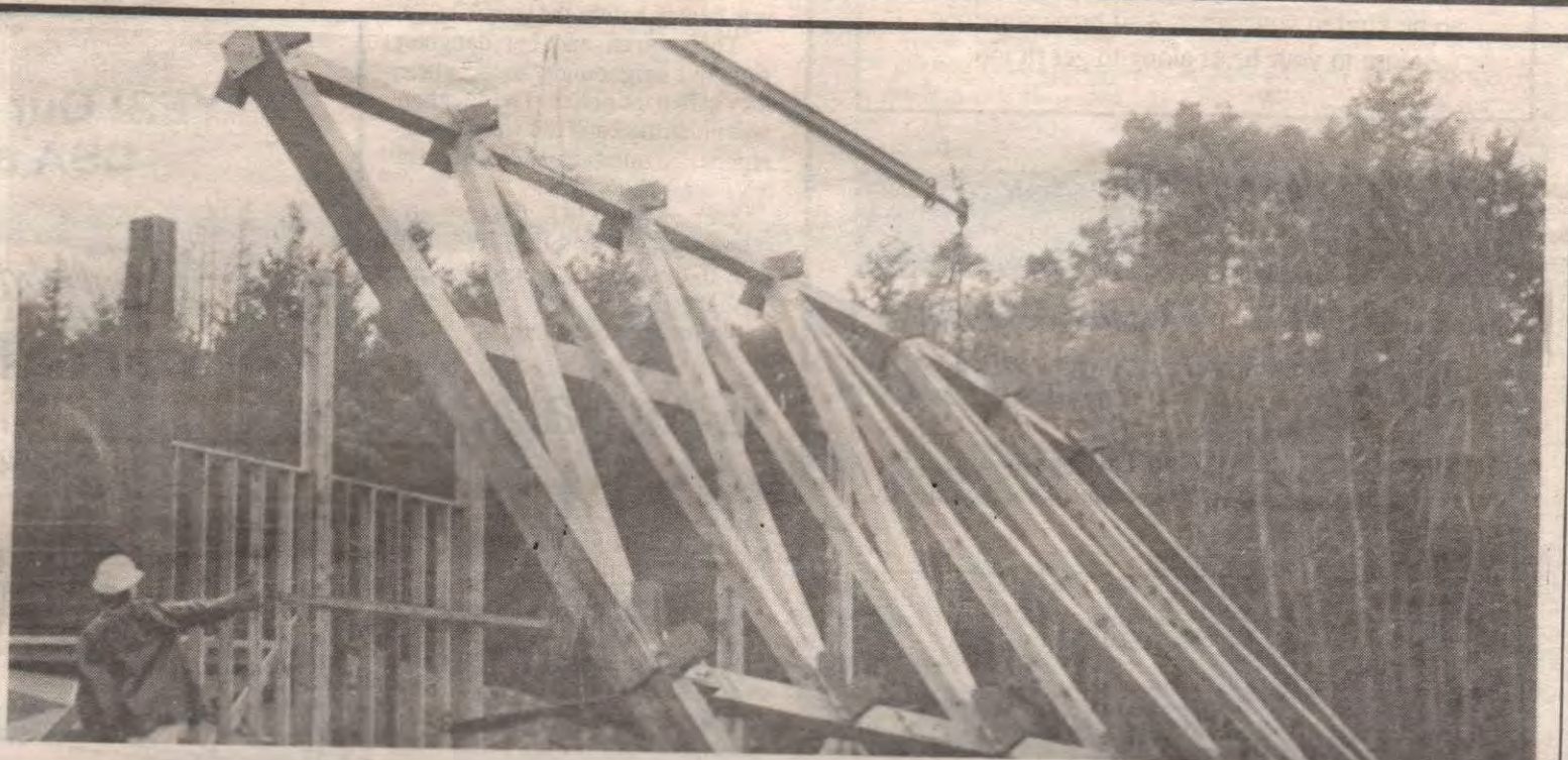
ON ITS WAY UP: ArtSpring's first wall was erected by crane power last Friday morning and the structure has continued to take shape since then. Island Arts Centre Society members say the building should be complete in time for this summer's Festival of the Arts.
