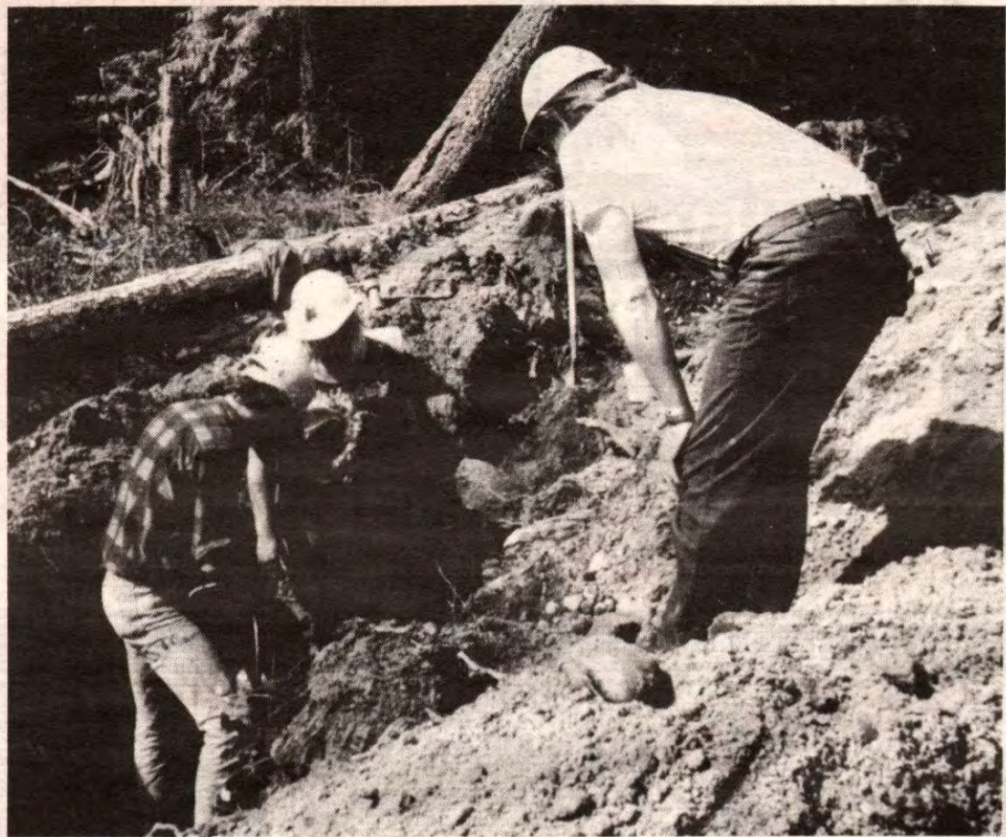
DIG IT: Workers with Hyland Excavating dig on McCoskrie Road for B.C. Tel's fibreoptics cable. First, a backhoe digs and moves pipe into place. Pipe is then welded to its neighbour and the backhoe re-covers it.
