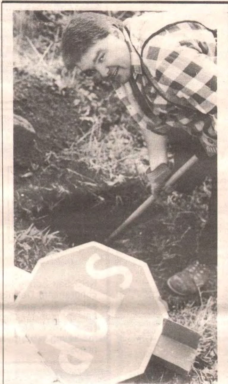
STOP IT!: Gord Hollingsworth of Victoria Highways Maintenance Corporation repairs results of hit and run sign bashing.
