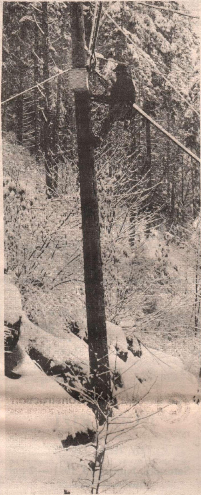
UP-GRADING: A B.C. Telephone lineman let his fingers do the working as he upgraded the system on Cranberry Road last week.
