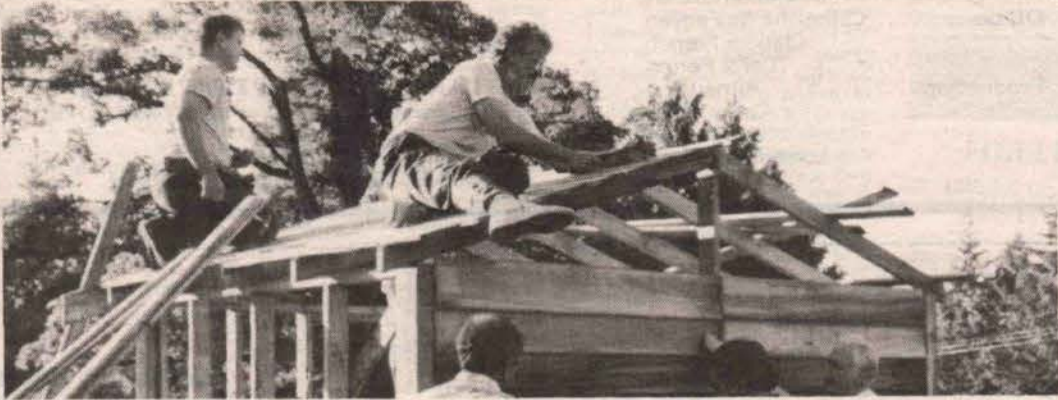
MEN AT WORK: Rotary Club members gave two evenings of skilled labour to the Community Society's pre-school building a storage shed last week. Pictured here (left to right) are Chris Bomford, Tony McEwen, Barry Cooke, Ron Smith and Don Harrison.
