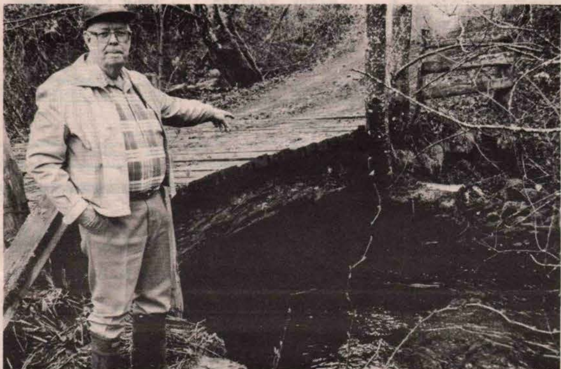
WASHED OUT: Ted O'Sullivan points to eroding bank of Fulford Creek which threatens the stability of a bridge on his property. O'Sullivan blames clear-cut logging on hills above Ford Lake as the source of his problem.
