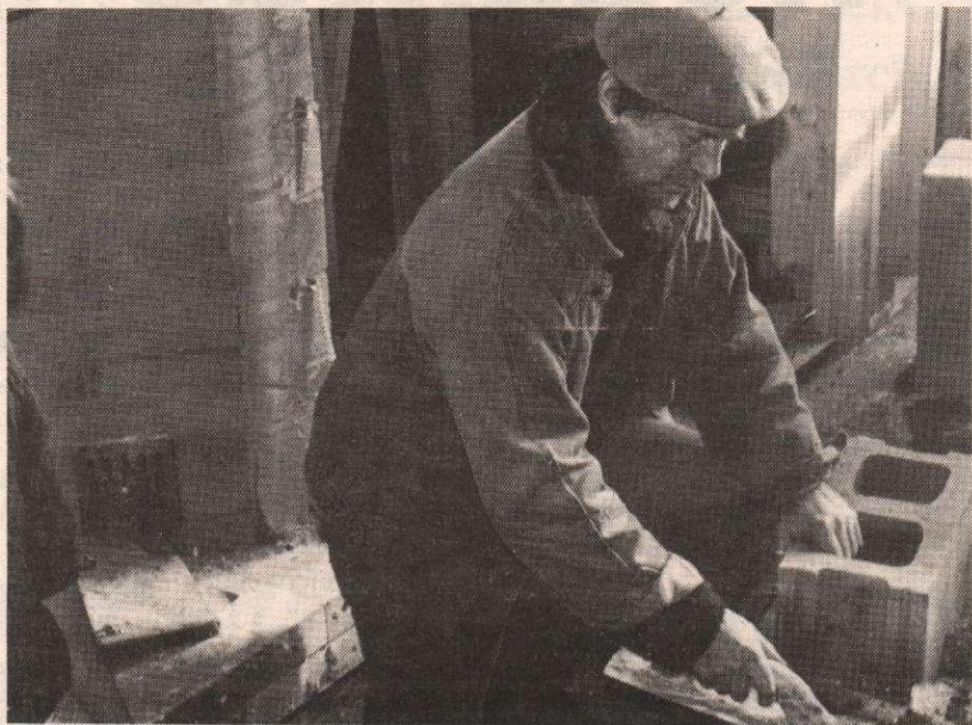
FIREPLACE CONSTRUCTION: Paul Hart works on the Rumford fireplace at Beaver Point Hall.
