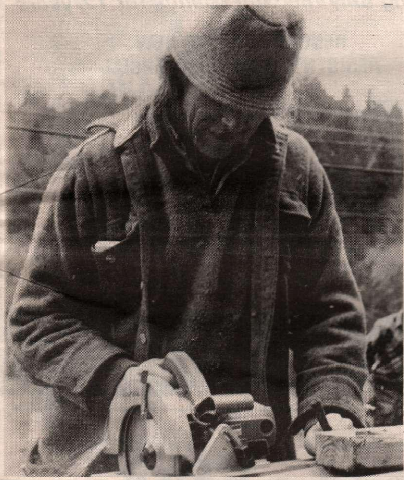
CONSTRUCTION: Island contractor Steve LaFortune (above) uses a cross-cut saw to cut a piece of siding for an outside covering at a Reginald Hill job site. At side, volunteer worker Doug Motherwell donates time at Beaver Point Hall renovation site. Springtime photos by Derrick Lundy
