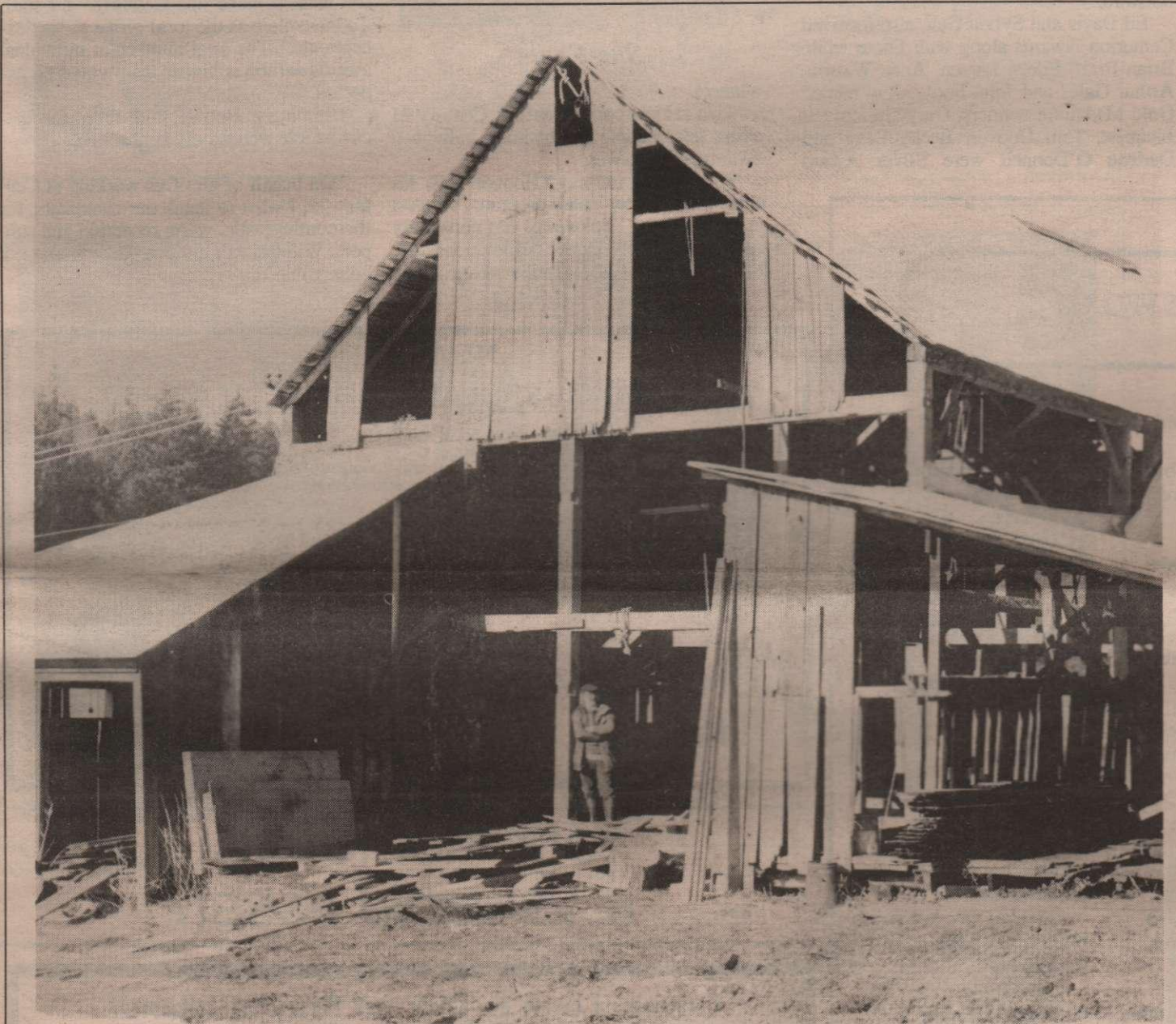
Jonathan Yardley heads up a restoration projection at the Henry Ruckle Barn at Ruckle Park
