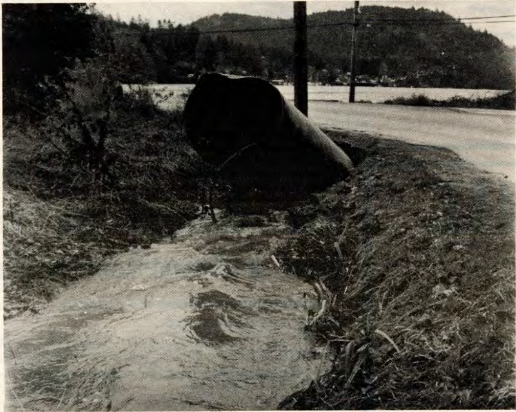
RAINED OUT - An avalanche of water forced this culvert in Fulford right out of the ground on Tuesday morning. Heavy rains the night before also washed out a portion of Burgoyne Bay Road.
