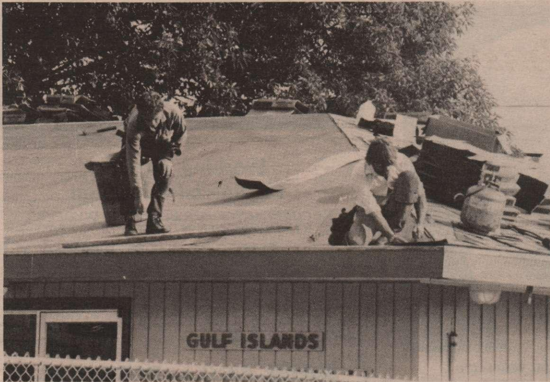
ON TOP OF THINGS: Workers recently spent a few days roaming overhead, giving Gulf Islands School District employees a new roof for the pending rainy season. The improvement is part of a series of upgrades made to the school board office this year.
