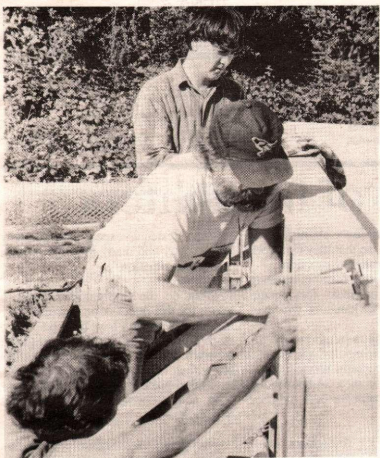
Work on the Salt Spring swimming pool continues in preparation for a test run at the end of the month. Putting up the strut supports (left to right) are: Bruce Mills, Richard Magnuson and Tom McKeachie. Members of the pool group are looking for volunteers to help complete the job. Driftwood photo by Bill Webster
