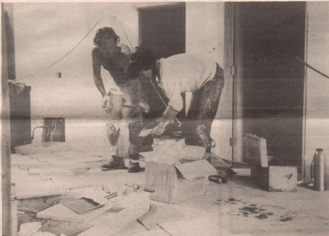
Jane Stack and Don Seed prepare to lay tiles at a Salt Spring Island home under construction. The headphones help cut down on the noise created when the tiles are cut.
