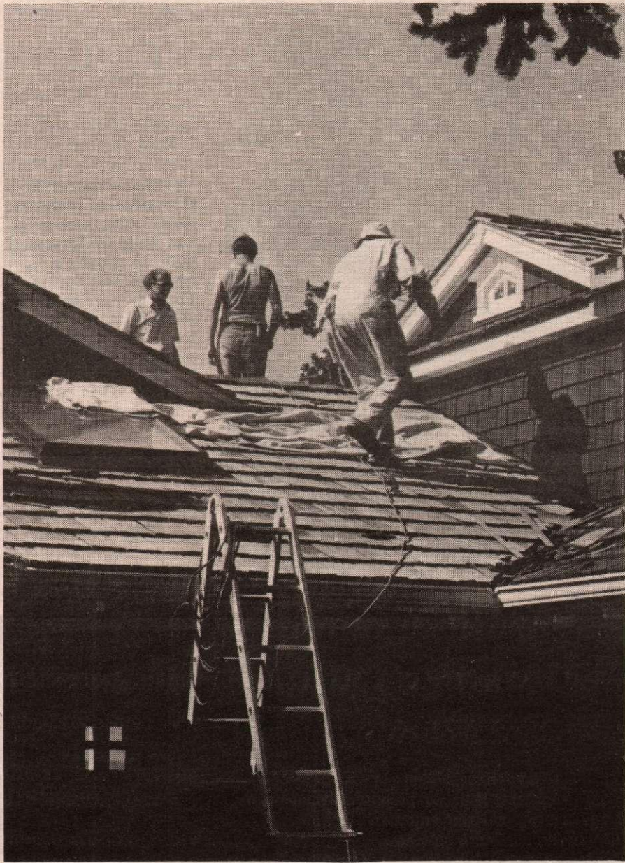
As well as replacing singles on the roof, these three workers installed a skylight on the left and painted parts of the house. They use a drop cloth and wear coveralls when painting. Note the ladder is not placed against the eaves trough, thereby preventing damage.
