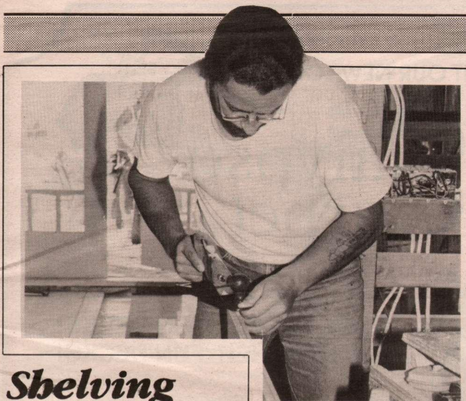
Carpenter Barry Manz planes off a piece of maple flooring for a tight fit. Local tradesmen are busy with new buildings, renovations and additions.
