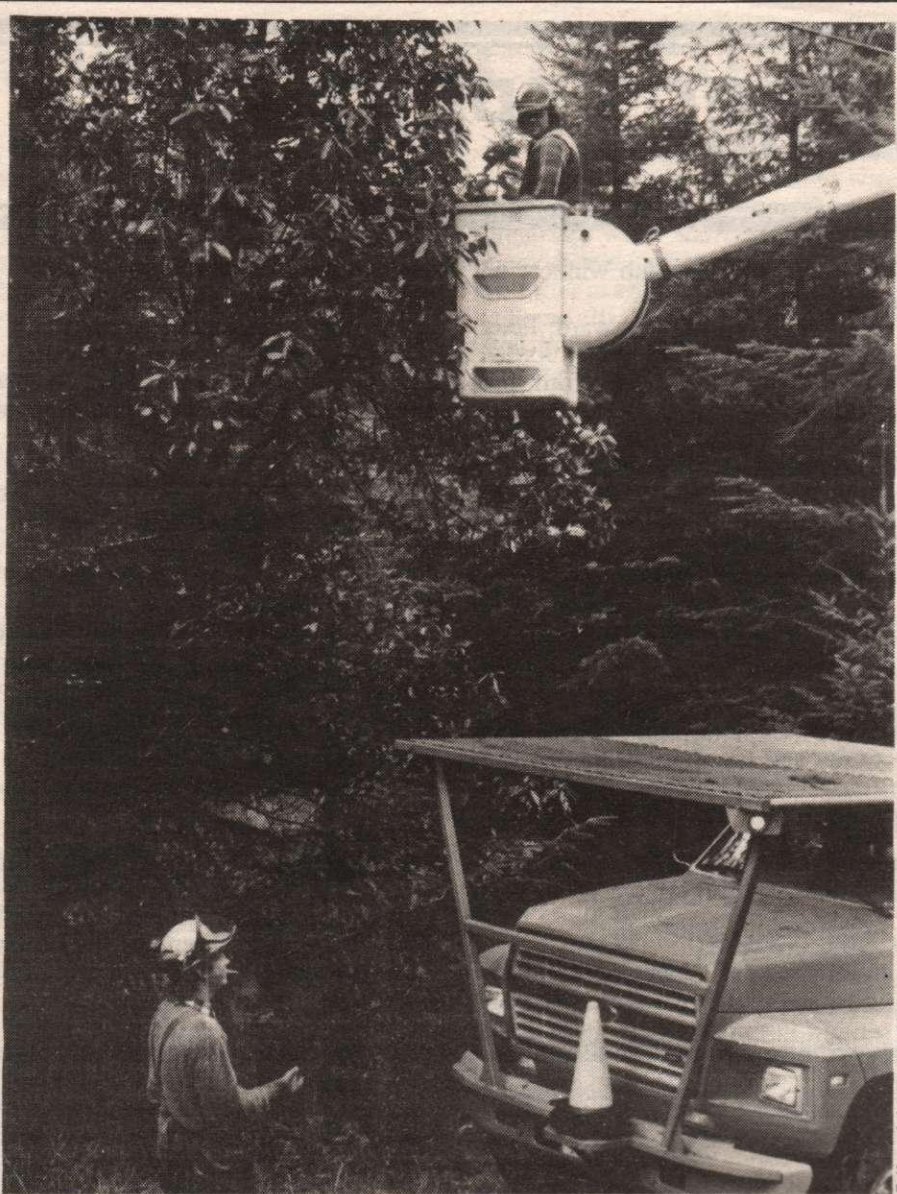
Overgrowth on Pender Island is cut back from wires
