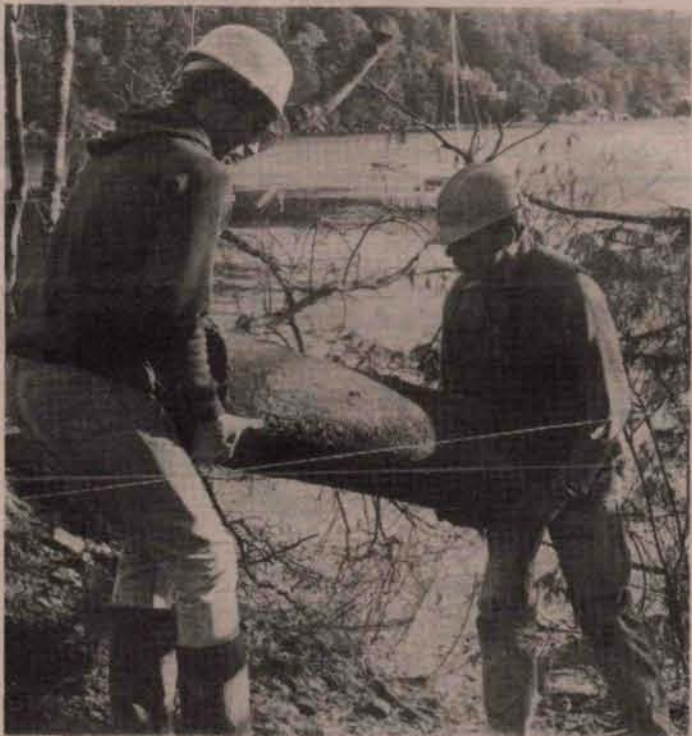
Construction on portions of the Ganges seawalk got underway in 1989 and continued throughout the year.
