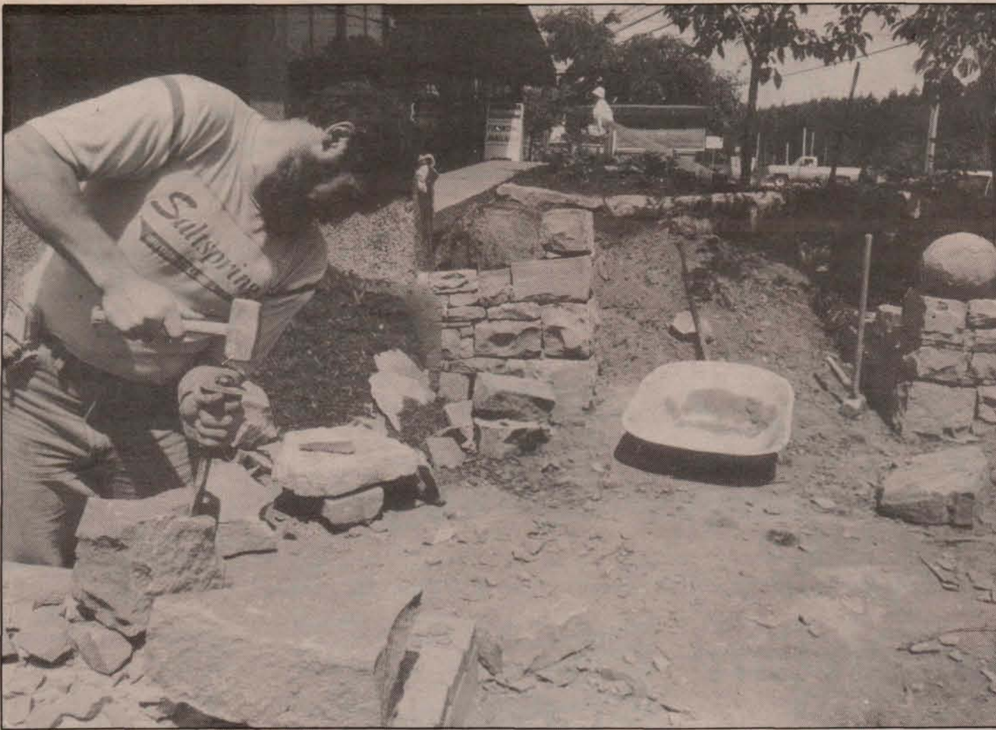
Salt Spring stonemason Andrew Currie worked last week to construct new entrance stairs at Island Savings Credit Union building in downtown Ganges. Project puts stairs through what was once a rock wall, increasing the number of main access paths to the building's front door.
