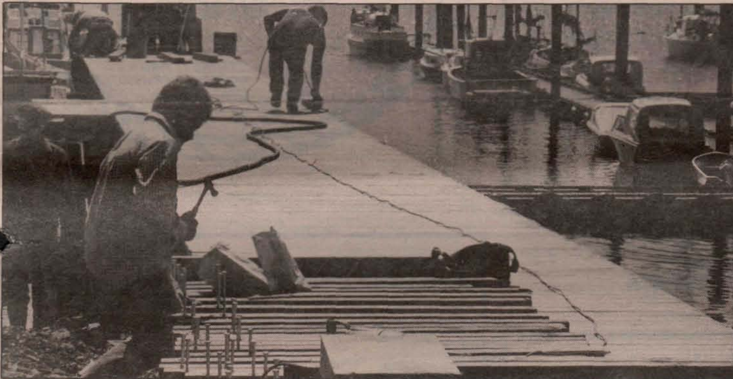
Redevelopment of Harbour's End marina began last week with installation of new walkway to floats (above). Design is to be in keeping with style of Ganges Harbour seawalk, to ensure conformity if it ever extends as far as marina. Other
