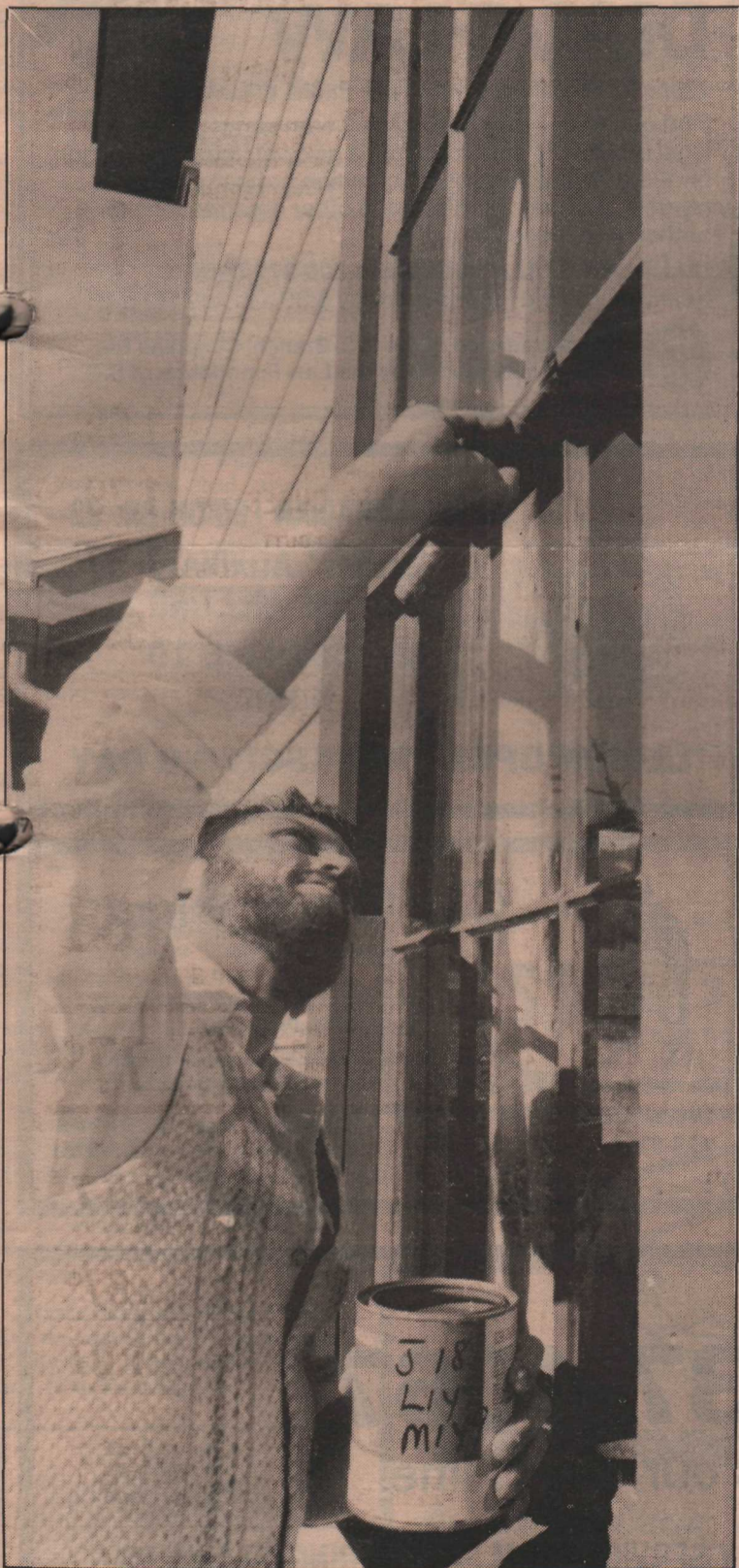
Bruce Whelan applies finishing coat of paint to window of historic farmhouse built by Henry Ruckle. Month-long restoration project was recently completed on Ruckle Park building.
